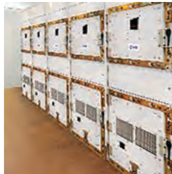
Medium Voltage Switchgear
