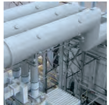
Medium Voltage Bus Duct
