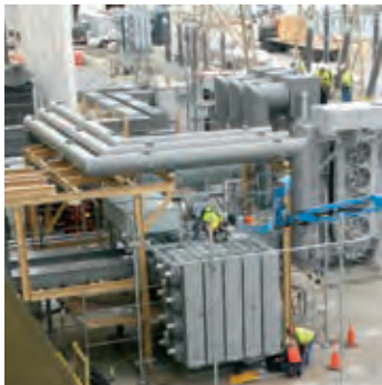
High Voltage SF 6 Bus Duct
