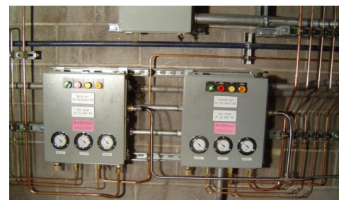
Dry air equipment installed at customer
