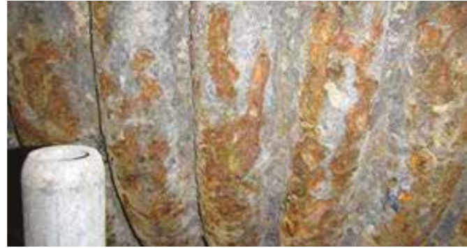
Fireside corrosion in a coal-fired boiler
