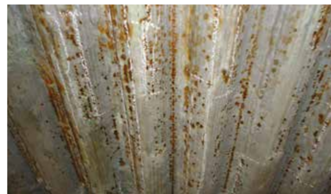
Waterwall after copper sulfate test
