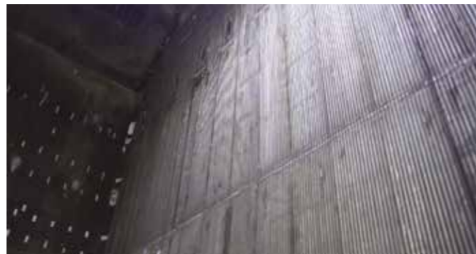
The AZZ WSI repair with Unifuse 622 extended the lifetime of the coal-fired boiler
