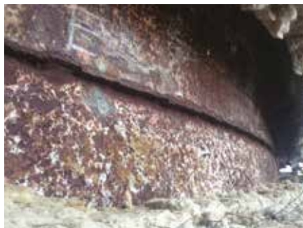
Full circumferential skirt cracks
