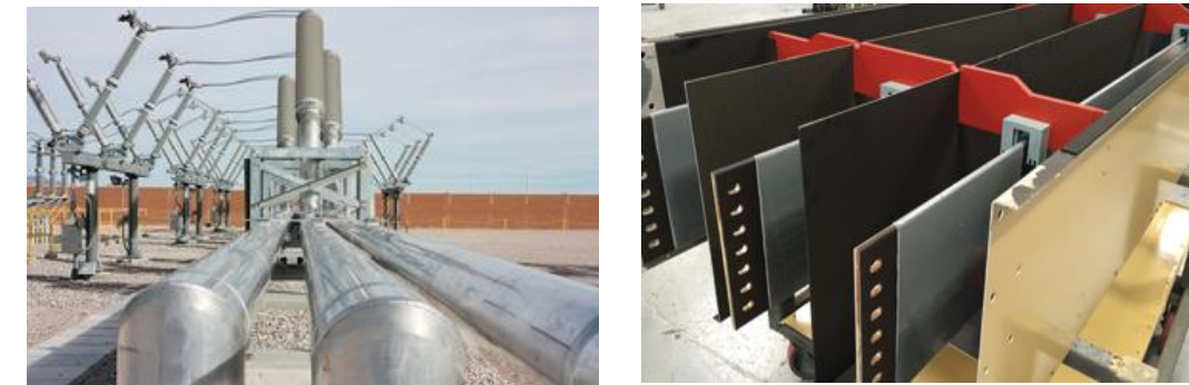
High Voltage Bus
